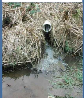
Illicit Sewer Discharges
